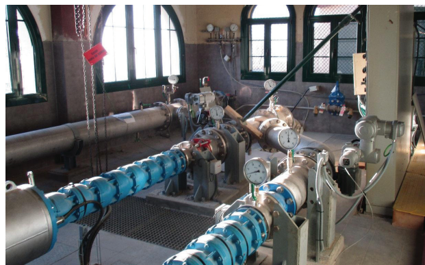
Figure 1 - Tibidabo Pumping Station
