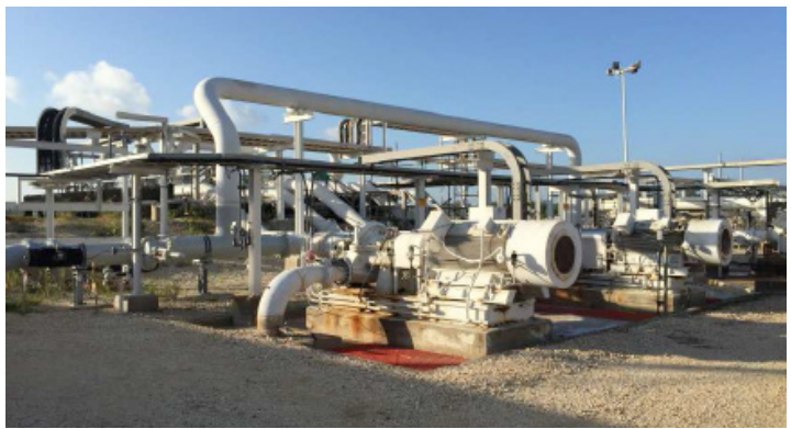
Figure 4 - Horizontal pumps maintain pressure in caverns and clarifier wells
