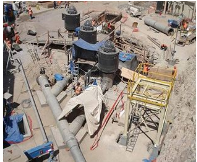
Toquepala Copper Mine electrical wiring frame and excavations for pipelines and bank boxes
