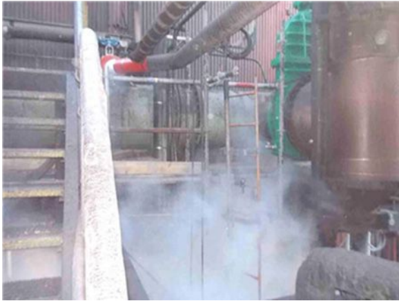
Existing coke oven gas piping
