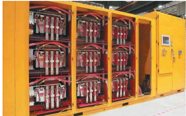
Fig. 3. EVSD Cabinet (Courtesy Siemens-Robicon)
