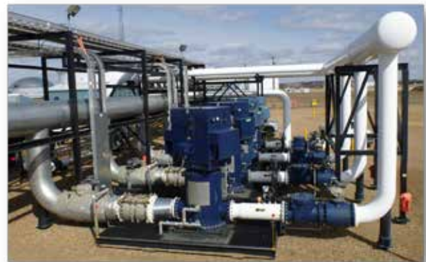
Figure 1 - Crude oil booster pump system
