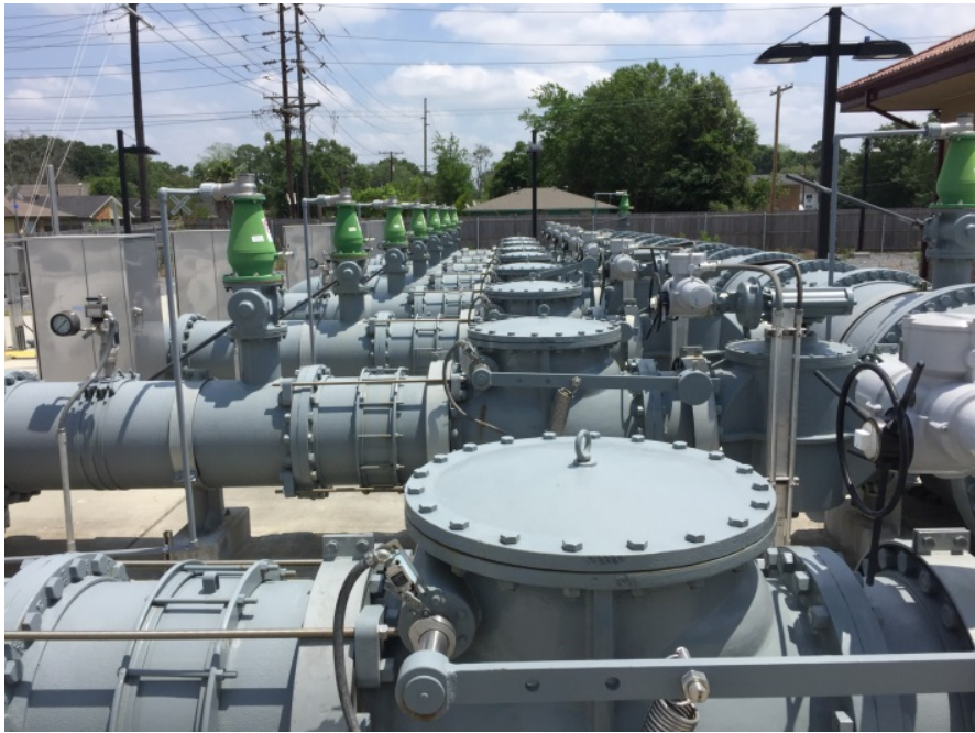
Figure 7: Vacuum breaker valves (in green, at left) at pump discharges.
