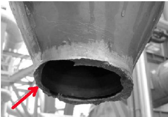
High transient forces fail reducer connection.
