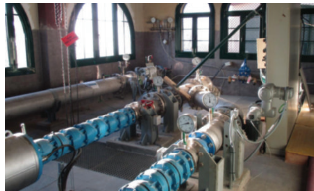
Figure 1 - Tibidabo Pumping Station
